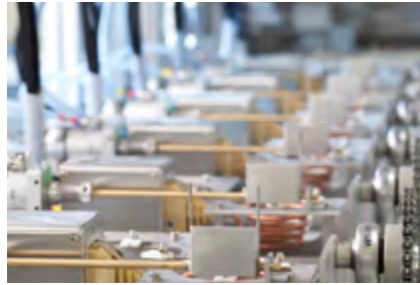
Row of fusion units ready for operation.
