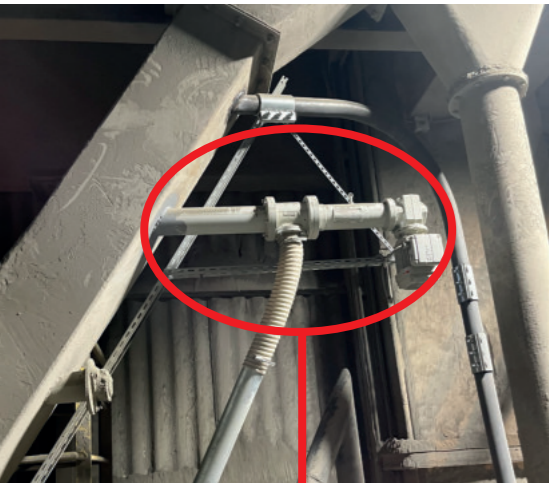
Installed Screw Sampler
